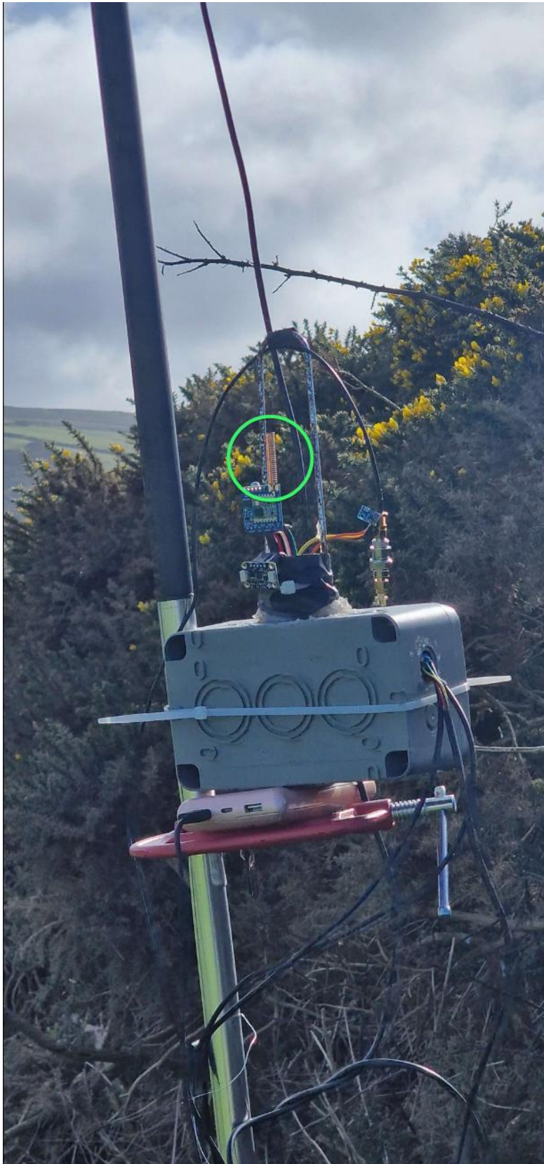
Appendix 2C – Weather station using a spring antenna (encircled green)
